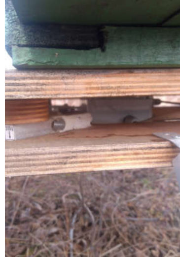
Fig. 7.14 Detail: insufficiently protected plywood.
